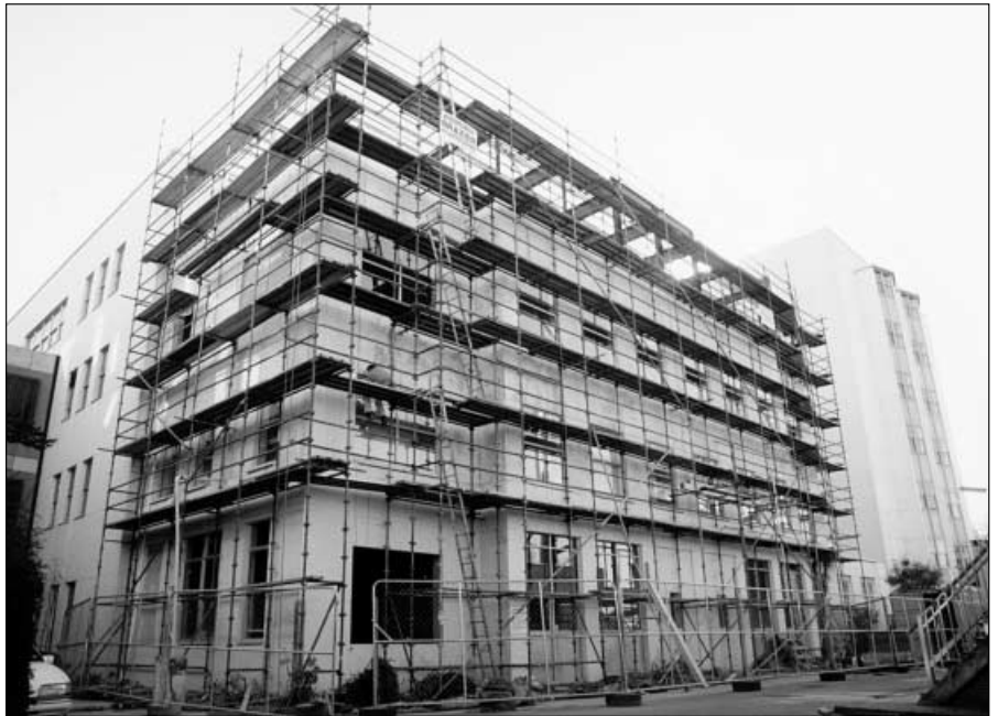
The new building which will accommodate the CAA, the second MRI and CT scanners, a new Gastrosocopy/Endoscopy Unit, Orthopaedic Outpatients and Paediatric offices.
