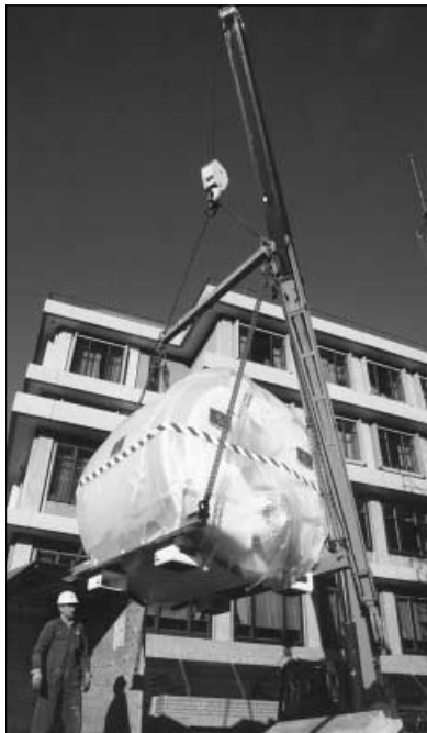
The magnet which is part of Radiology's new scanning facilities is lifted into the building.
